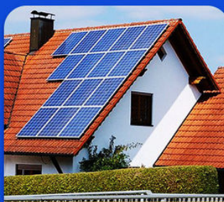
Solar Energy Storage
