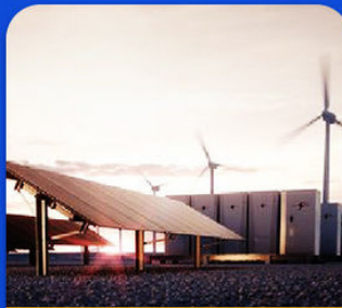
Industrial & Commercial energy Storage
